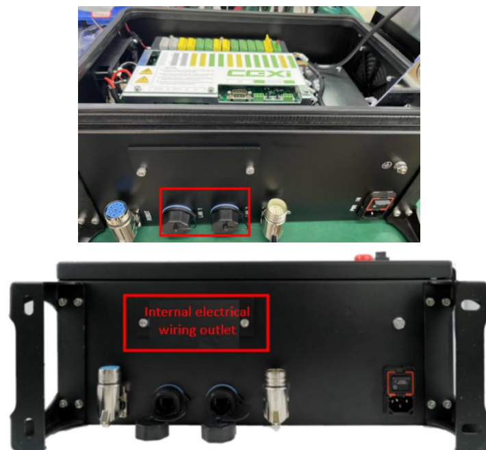
Figure 78 Internal interface of the control cabinet
