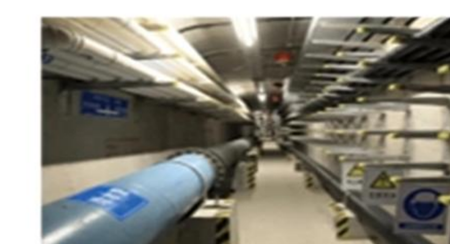
Pipe gallery tunnel operation
