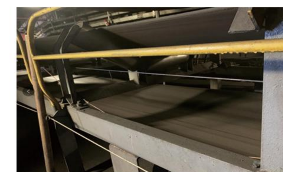
Bottom of belt conveyor line
